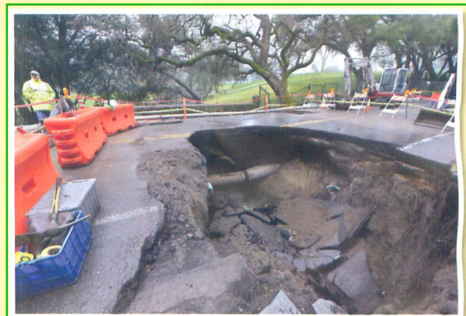
Miner Road Sink Hole in Orinda
